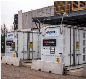
C&I BESS Projects
