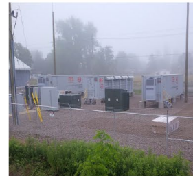
Strathroy BESS Facility
