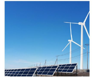
Arviat Microgrid Facility
